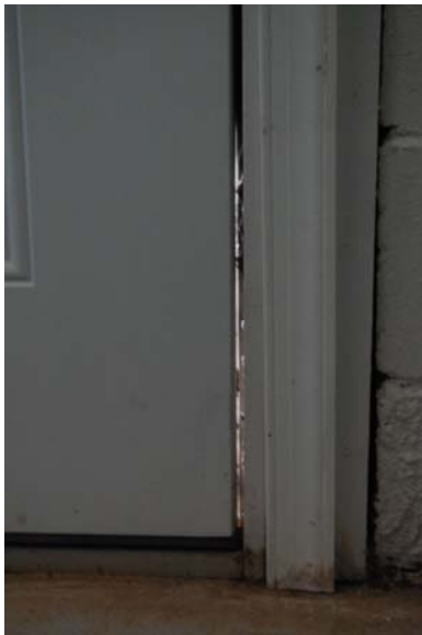
Bad Air Leak!
